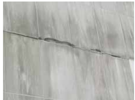
Masonry used on the exterior of modern buildings is generally a cladding attached to a separate structure. Clips, anchors or shelf angles are used to attach the stone panels or brick masonry. The deterioration of these anchors is an area of potential deterioration and failure. Monitoring the condition of these anchors is a vital part of a maintenance plan, as their failure can lead to very significant damage.
