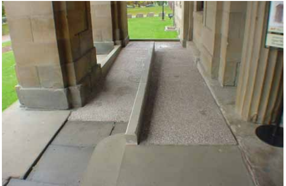
Adding a ramp to meet accessibility requirements should be designed to be compatible with a building's character. This new ramp at Province House in Charlottetown was discretely integrated into one side of an existing entrance porch.
