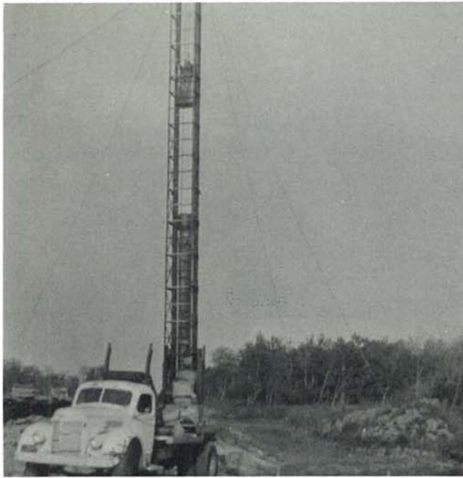
Bunio Pile Driver, this equipment was built by John Bunio, working at Catfish creek near Fort Alexander.
