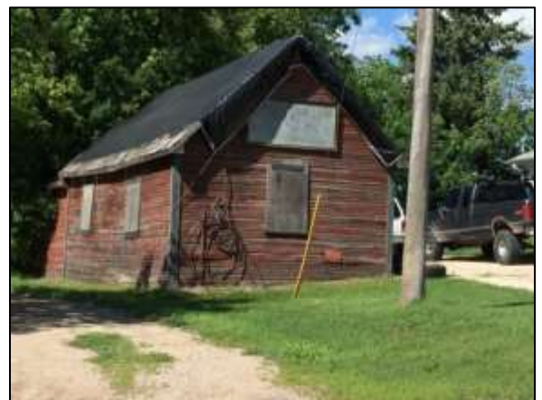
The Domke Blacksmith Shop, is one of the last remaining older buildings in the village
