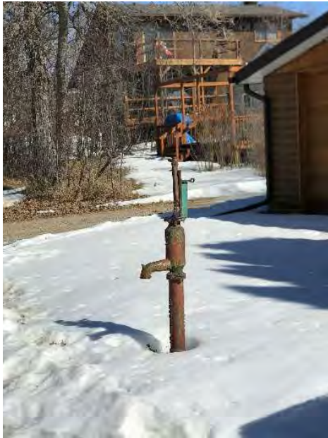
Typical water pump
