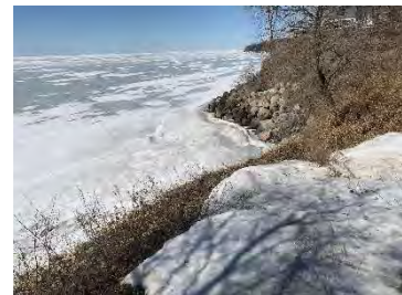
Note the erosion here – loss of cliffside and attempt to stop erosion with large boulders
