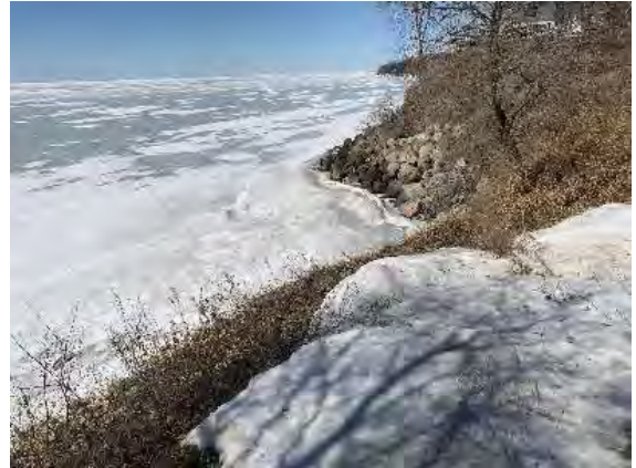
View of erosion on Grand Marais shoreline, just west of Grand Marais Boulevard South. Note the use of large boulders to try and stabilize the cliff bank.
