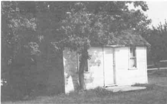
155) Summer Kitchen Construction Date: ca. 1910 Location: SE 27-15-6E Present Owner: R. Krahn Present Use: Storage Construction: walls - horizontal siding on milled wooden frame roof - wood shingles on milled wooden rafters Integrity: Unaltered Condition: Good
