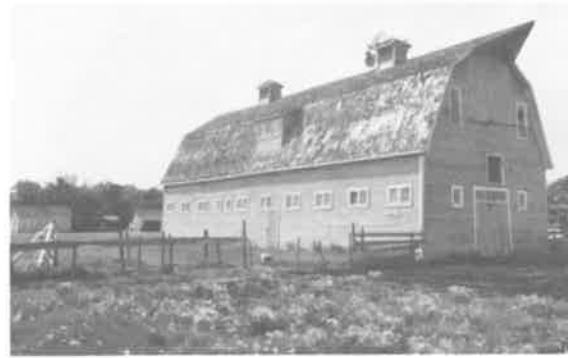
104) Large Light Wood Frame Barn Construction Date: 1915 Location: SE 1-15-4E Present Owner: Mr. Macklin Present Use: Functioning Barn Construction: walls - horizontal siding on milled wooden frame roof - wood shingles on built-up wooden rafters Integrity: Unaltered Condition: Good
