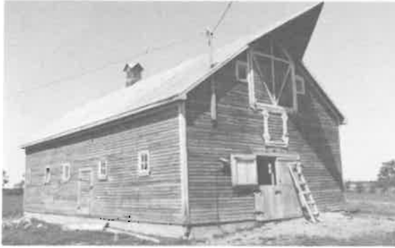
109) Large Light Wood Frame Barn Construction Date: ca. 1920 Location: NE 18-16-8E Present Owner: G. Lloyd Present Use: Functioning Barn Construction: walls - horizontal siding on milled wooden frame roof - metal sheeting on milled wooden rafters Integrity: Unaltered Condition: Good
