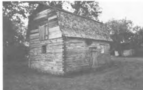
108) Log Barn Construction Date: ca. 1920 Location: Libau Present Owner: Present Use: Storage Construction: walls - squared dovetailed logs roof - wood shingles on milled wooden rafters Integrity: Unaltered Condition: Fair
