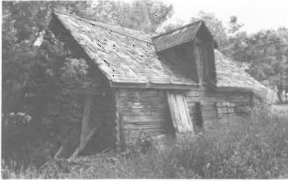
129) Log Granary Construction Date: ca. 1920 Location: River Lot #277 Present Owner: Nick Switski Present Use: Abandoned Construction: walls - dovetailed logs roof - wood shingles on milled wooden rafters Integrity: the gabled dormer was added to accept grain from an auger Condition: Fair
