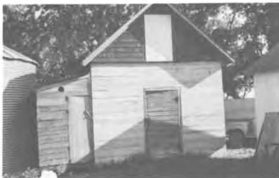
159) Ice House Construction Date: ca. 1910 Location: NW 24-15-6E Present Owner: C. Horbady Present Use: Storage Construction: walls - solid poured concrete roof - asphalt shingles on milled wooden rafters Integrity: Unaltered Condition: Good
