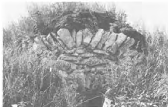
160) Root Cellar Construction Date: ca. 1920 Location: SE 2-13-5E Present Owner: Present Use: Abandoned Construction: walls - fieldstone barrel vault roof - fieldstone, covered with sod Integrity: Unaltered Condition: Poor
