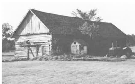
112) Log Barn Construction Date: ca. 1925 Location: SW 13-15-6E Present Owner: Mr. R. Ozol Present Use: Storage Construction: walls - squared dovetailed logs roof - wood shingles on squared logs Integrity: Unaltered Condition: Fair
