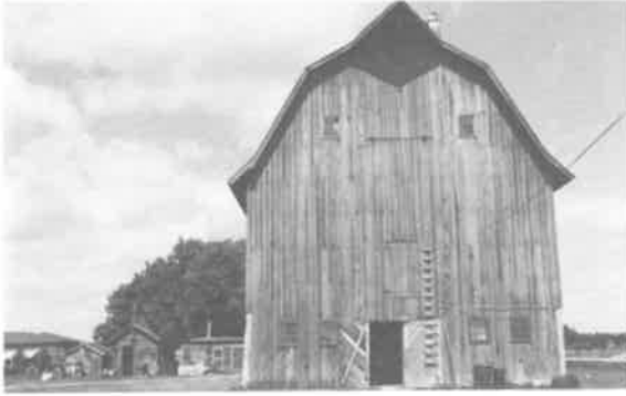
101) Large Light Wood Frame Barn Construction Date: 1912 Location: River Lot #20 Present Owner: Mr. Overwater Present Use: Storage Construction: walls - concrete stable and light frame loft roof - wood shingles on built-up wooden rafters Integrity: Unaltered Condition: Good Notes: This building is also discussed on pages 65-66.
