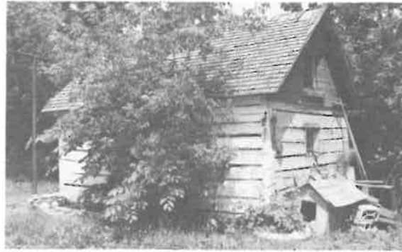
154) Summer Kitchen Construction Date: 1926 Location: River Lot #240 Present Owner: E. Huzarski Present Use: Storage Construction: walls - dovetailed logs roof - wood shingles on milled wooden rafters Integrity: Interior has been gutted Condition: Fair
