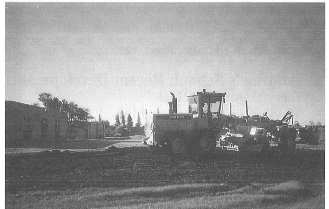
R.M. of St. Andrews equipment and operators working on the drainage plan.
