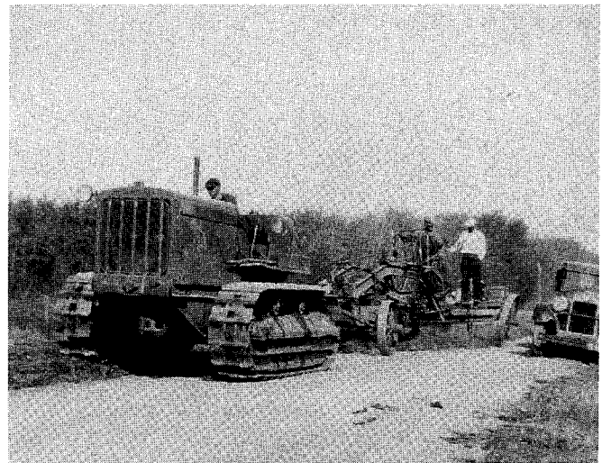
Municipal road building (contractor and operator unknown) undertaken in 1938 with mechanical equipment for the first time by the R.M. of St. Clements 1 1/4 miles north of Libau (21-15-6E) in front of the farm of Fred Wakshinski.
